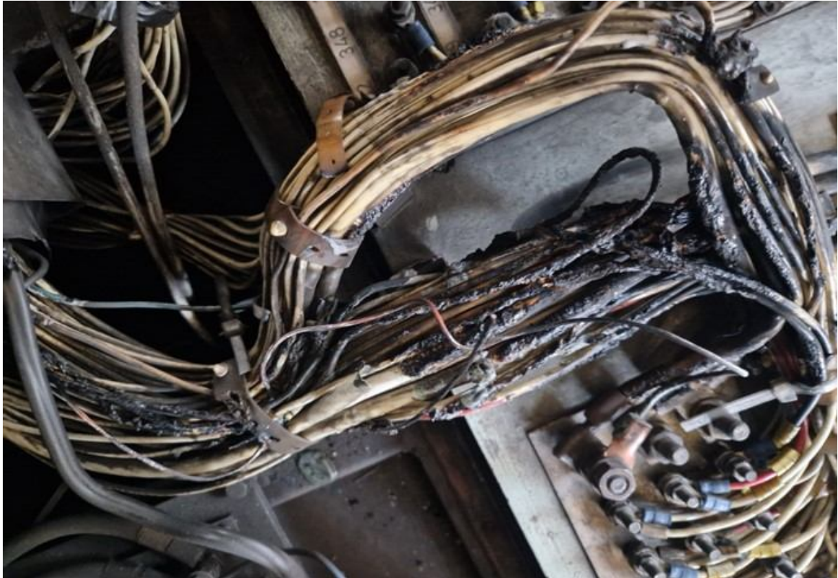
Fig. 4.16. Burnt cables on conductor 870
